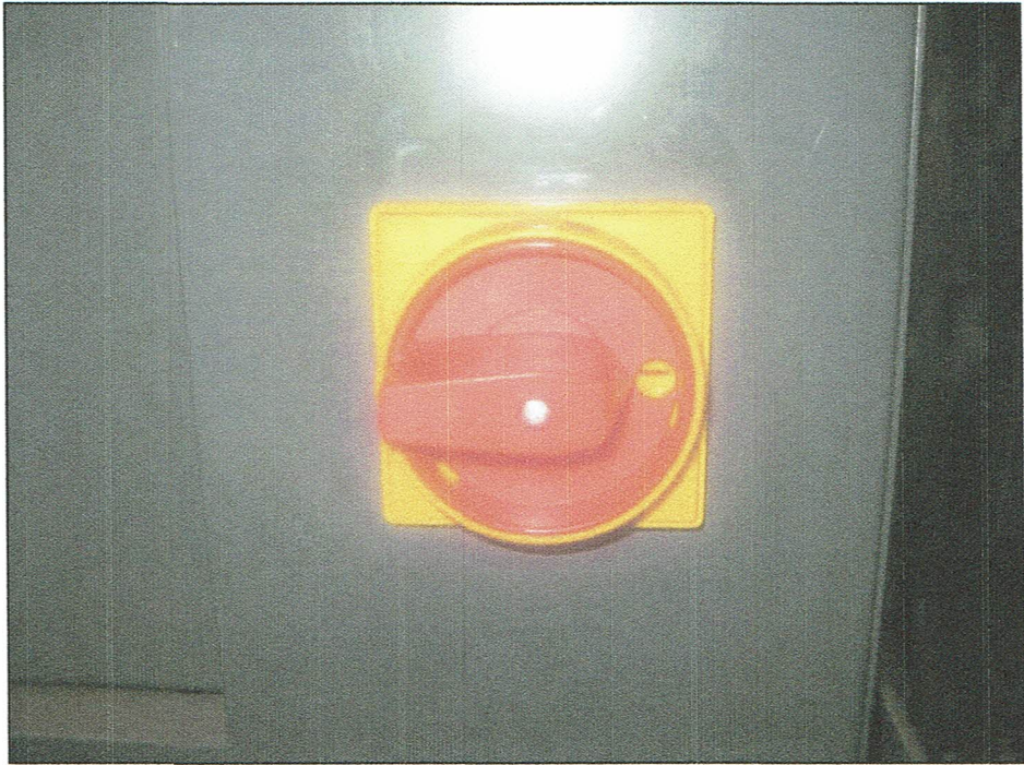
Photo 11: XEKL 455 MT: Lockable isolation switch
